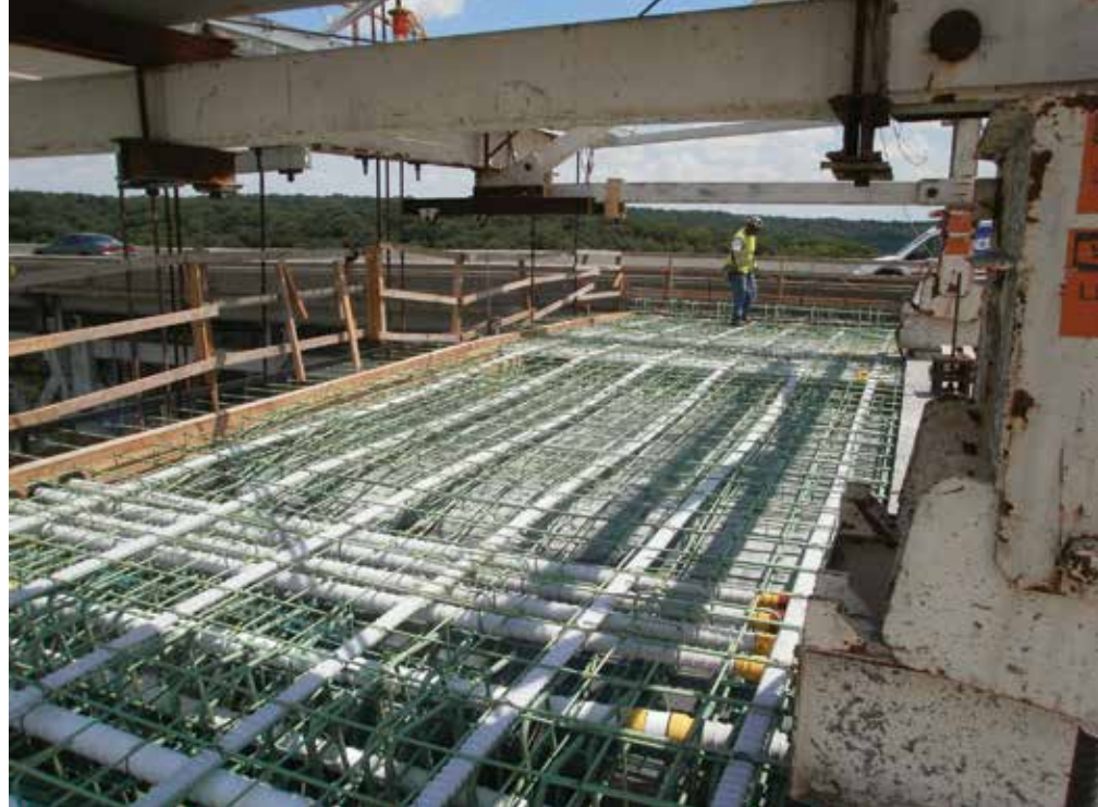
Transverse four-strand tendons in the top slab and longitudinal post-tensioning were used to achieve “zero-tension” criteria under service load conditions. Photo: Jeff Weiler, OmniPro Services.
