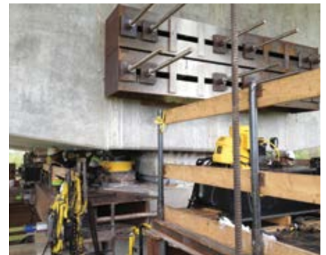
Transverse post tensioning of 2.5 million lbs to distribute jacking forces in the segment bottom slab.
