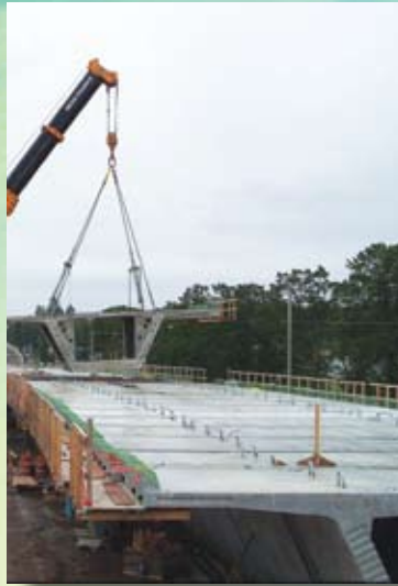
SW Line Bridge, Nalley Valley Interchange (Photo Courtesy of Guy F. Atkinson Construction, LLC)
