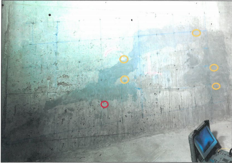
Figure 5: Photograph of Segment 2-1 overlaid with Impact Echo results. Yellow circles indicate questionable conditions, and red circles indicate poor conditions. The points that do not have circles are sound conditions. The horizontal measurements are measured from the south joint, which is the left side of the photograph.
