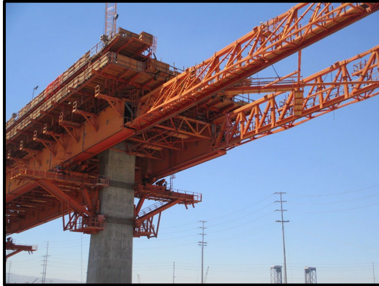
Long Beach International Gateway Bridge (Gerald Desmond Bridge Replacement), Long Beach, CA
