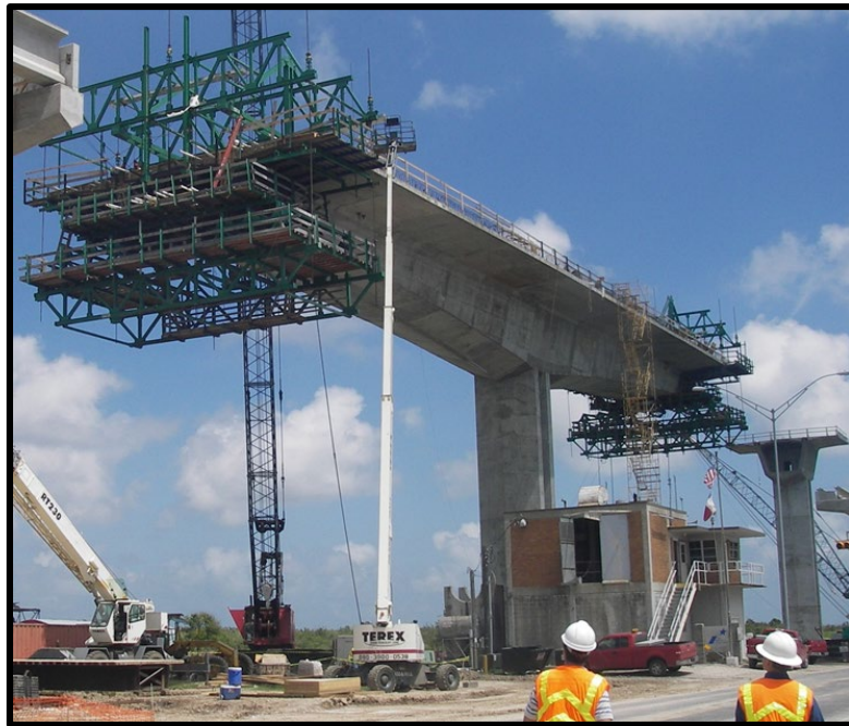
Cast-in-Place Balanced Cantilever the Gulf Intracoastal Waterway Bridge in Matagorda, TX (Photo Courtesy of ASBI)
