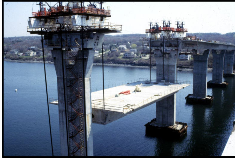
Lifting an Entire Span, Jamestown Verrazzano Bridge, RI (Photo Courtesy of FIGG Engineering Group)
