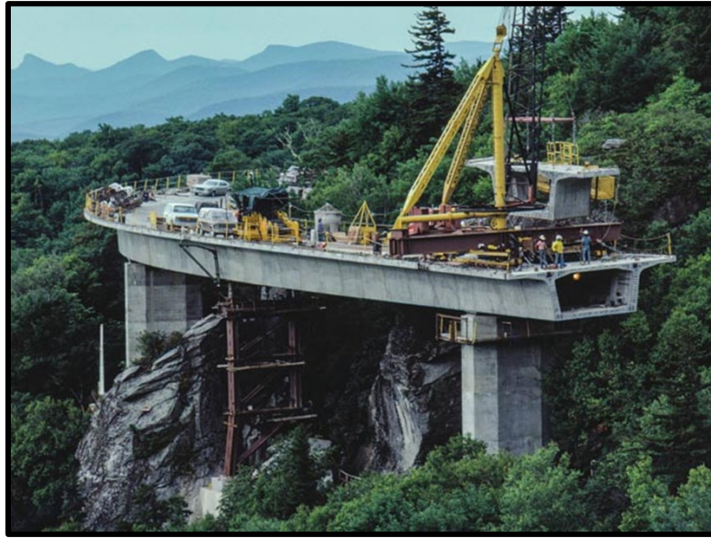
Progressive Placement, Linn Cove Viaduct, Blue Ridge Parkway, NC (Photo Courtesy of FIGG Engineering Group)
