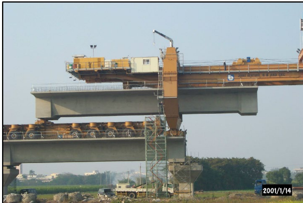
Figure 4-4. Launching of Full-Span Box Girder with Transporter and Overhead Gantry for Taiwan High-Speed Rail (Photo Courtesy of SYSTRA IBT)
