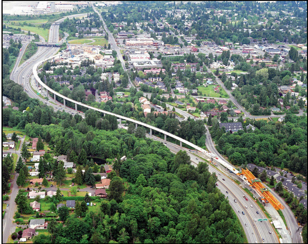
Figure 4-37. Overhead Gantry Erection of Sound Transit Box Girder Guideway in Seattle, WA (Photo Courtesy of SYSTRA IBT)
