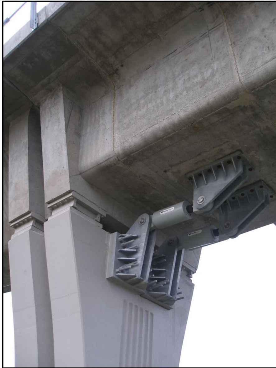
Figure 4-17. Shock Transmission Units (STUs) Connecting End of Guideway to Substructure on Sound Transit in Seattle, WA (Photo Courtesy of SYSTRA IBT)
