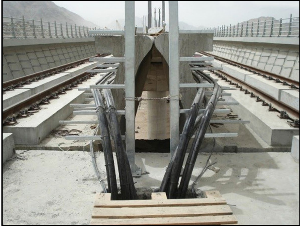
Figure 4-21. Transition of System Cabling from U-Section Parapet Through Opening in Adjacent Structure (Photo Courtesy of SYSTRA IBT)
