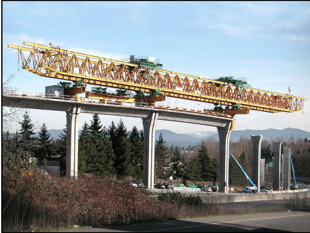
Figure 4-1. Span-by-Span Erection with Overhead Gantry of Sound Transit Box Girder Guideway in Seattle, WA (Photo Courtesy of SYSTRA IBT)
