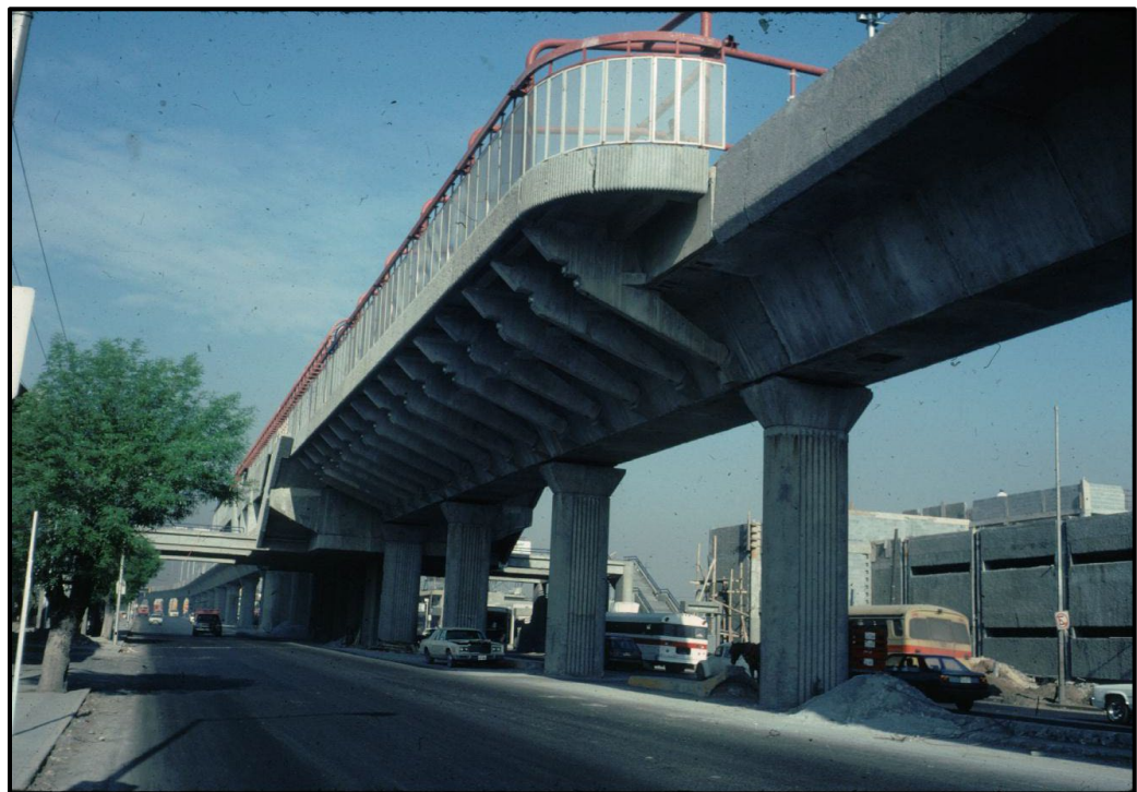
Figure 4-6. Station Platform Supported Directly by Box Girder for Metro of Monterrey in Mexico (Photo Courtesy of SYSTRA IBT)
