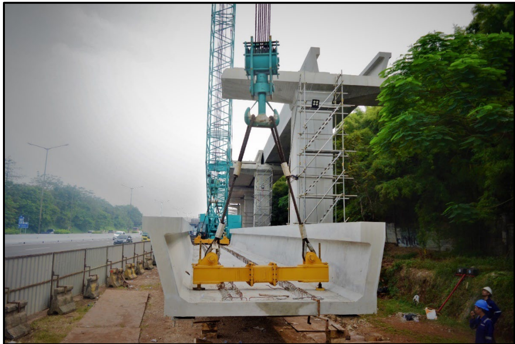
Figure 4-12. Full-Span Erection of Narrow U-Section Guideway with Cranes for Jabodebek Greater Jakarta LRT, Indonesia (Photo Courtesy of SYSTRA IBT)
