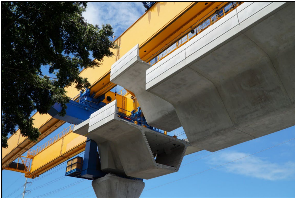
Figure 4-2. Span-by-Span Erection with Overhead Gantry of HART Box Girder Guideway in Honolulu, HI (Photo Courtesy of SYSTRA IBT)
