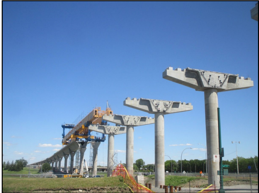
Figure 4-7. Hammerhead Bent Caps That Will Support Both the Station Platform and the Integral Box Girder Guideway for Réseau Express Métropolitain (REM) in Montreal, Canada (Photo Courtesy of SYSTRA IBT)
