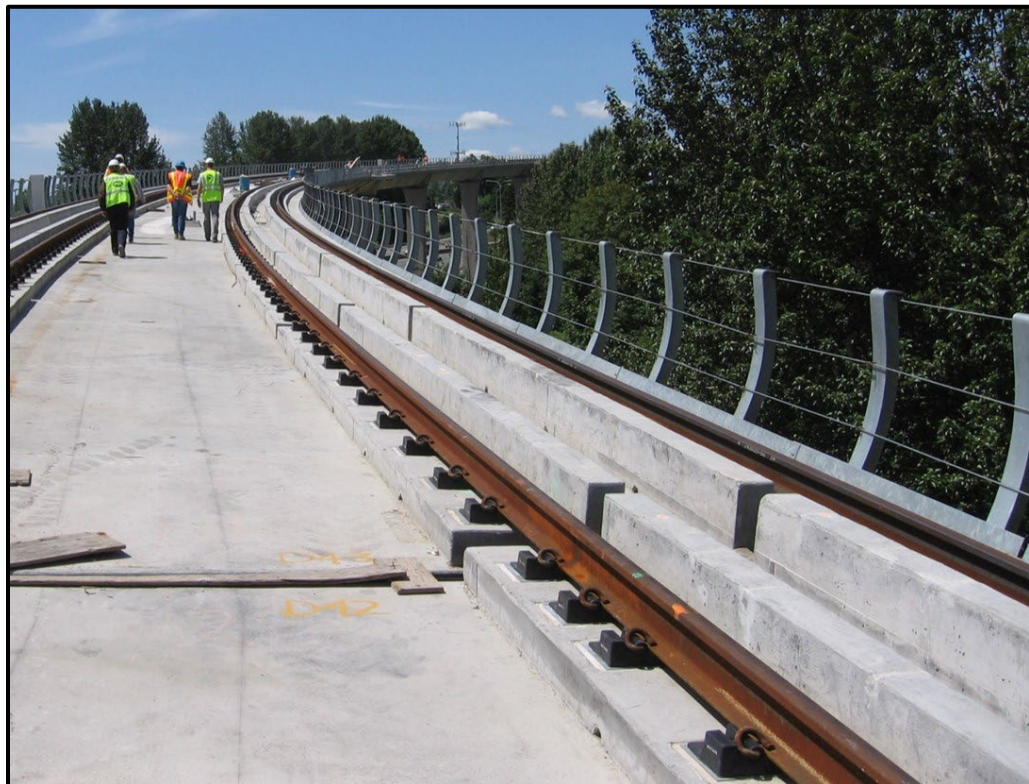
Figure 4-35. Direct-Fixation Rails Supported by Plinths on Sound Transit in Seattle, WA (Photo Courtesy of SYSTRA IBT)
