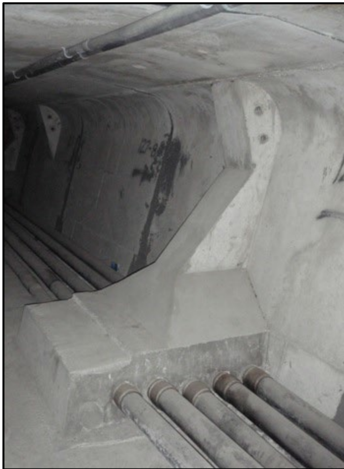
Figure 5-1. External Tendons and Deviation Block Inside a Box Section (Photo Courtesy of ASBI)
