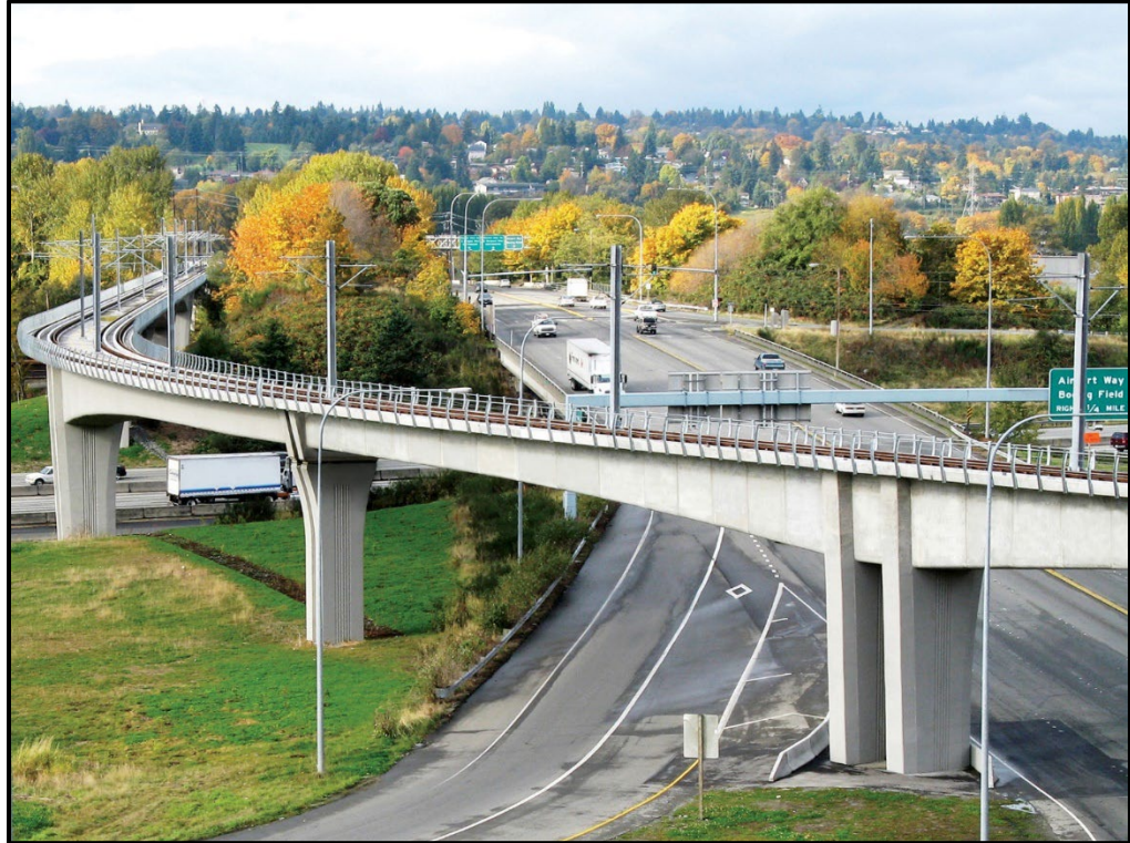
Figure 4-3. Long-Span Variable-Depth Box Girder with Structural Continuity at Piers for Sound Transit in Seattle, WA (Photo Courtesy of SYSTRA IBT)
