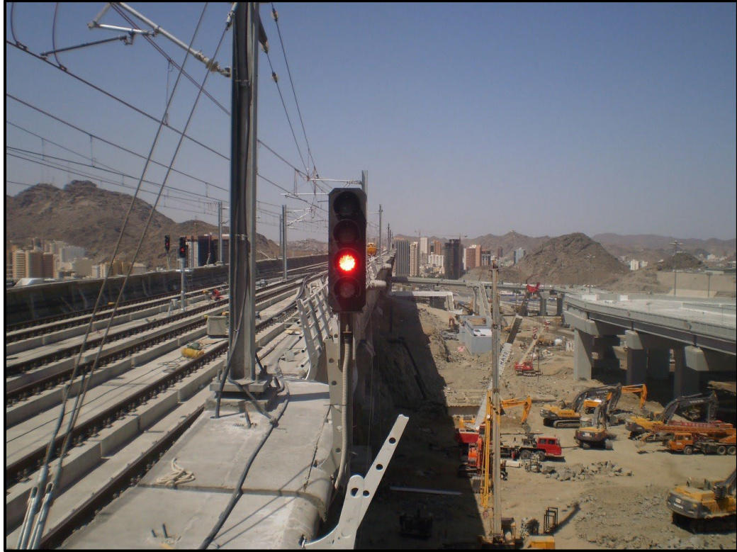
Figure 4-28. Signal Post Mounted to Segment for MMMP in Makkah, Kingdom of Saudi Arabia (Photo Courtesy of SYSTRA IBT)
