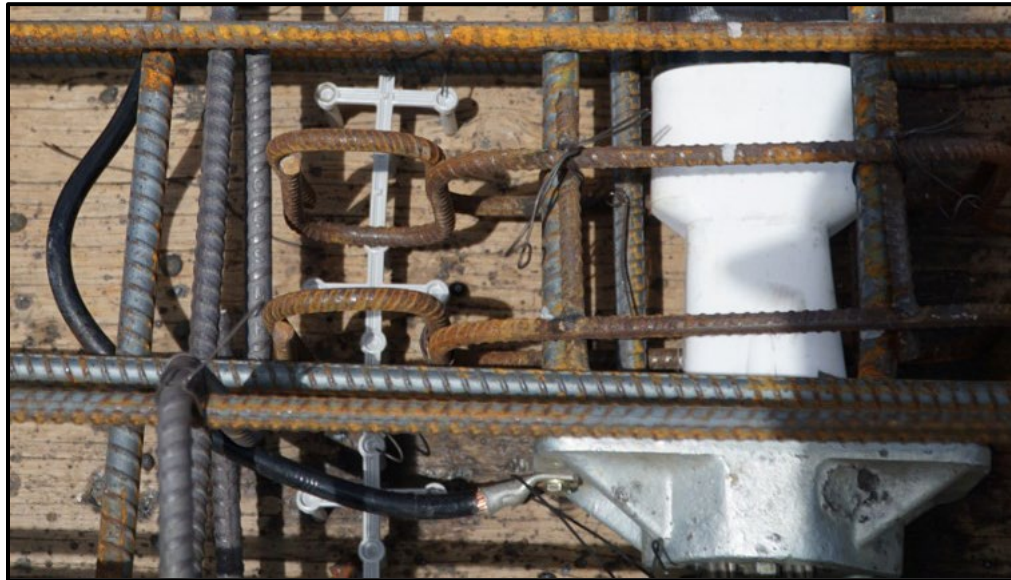
Figure 4-31. Bonding Detail for Transverse Post-Tensioning Anchor Head in Top Slab of Guideway (Photo Courtesy of SYSTRA IBT)
