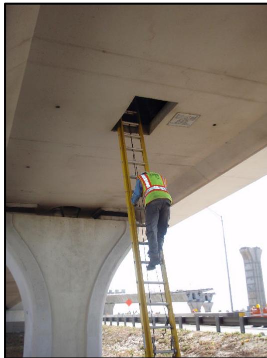
Figure 5-3. Bottom Slab Access Hatch Entered with External Ladder (Photo Courtesy of ASBI)
