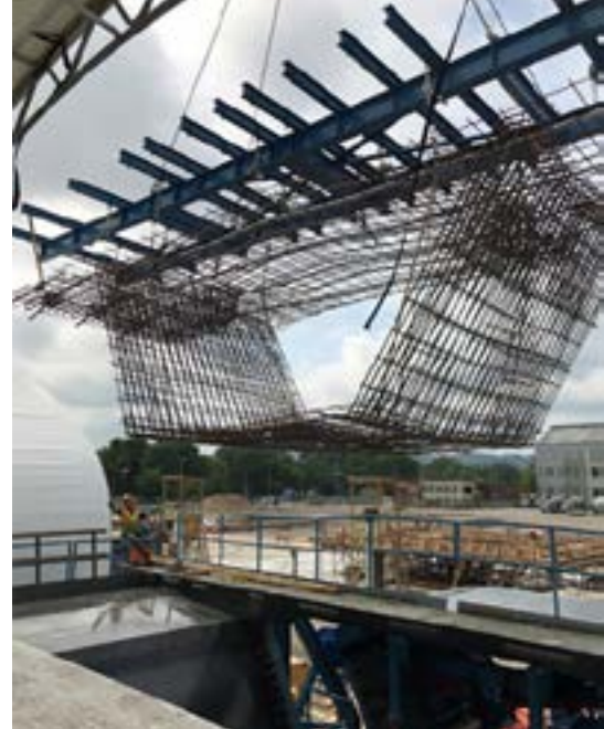
Reinforcing bar cage with transverse tendons being installed into forms. Photo: Johnson Bros.
