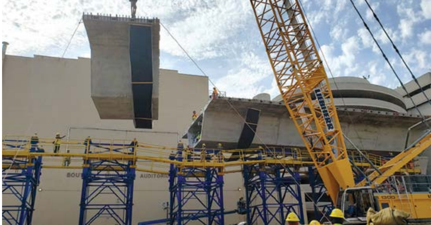
Erection of a precast concrete box-girder segment on temporary support towers for the first span of the central business district bridges. Photo: Volkert Inc.
