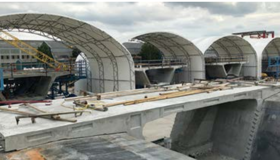
Casting cells for precast concrete box-girder segments with protective covers. Photo: Johnson Bros.
