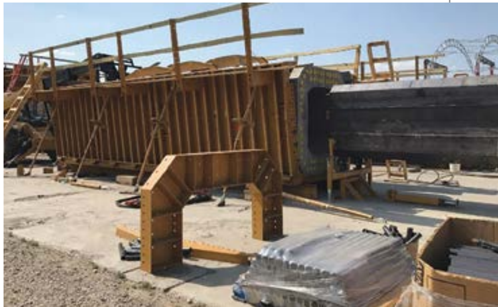
Precast concrete column in form with core form being extracted. Photo: Johnson Bros.
