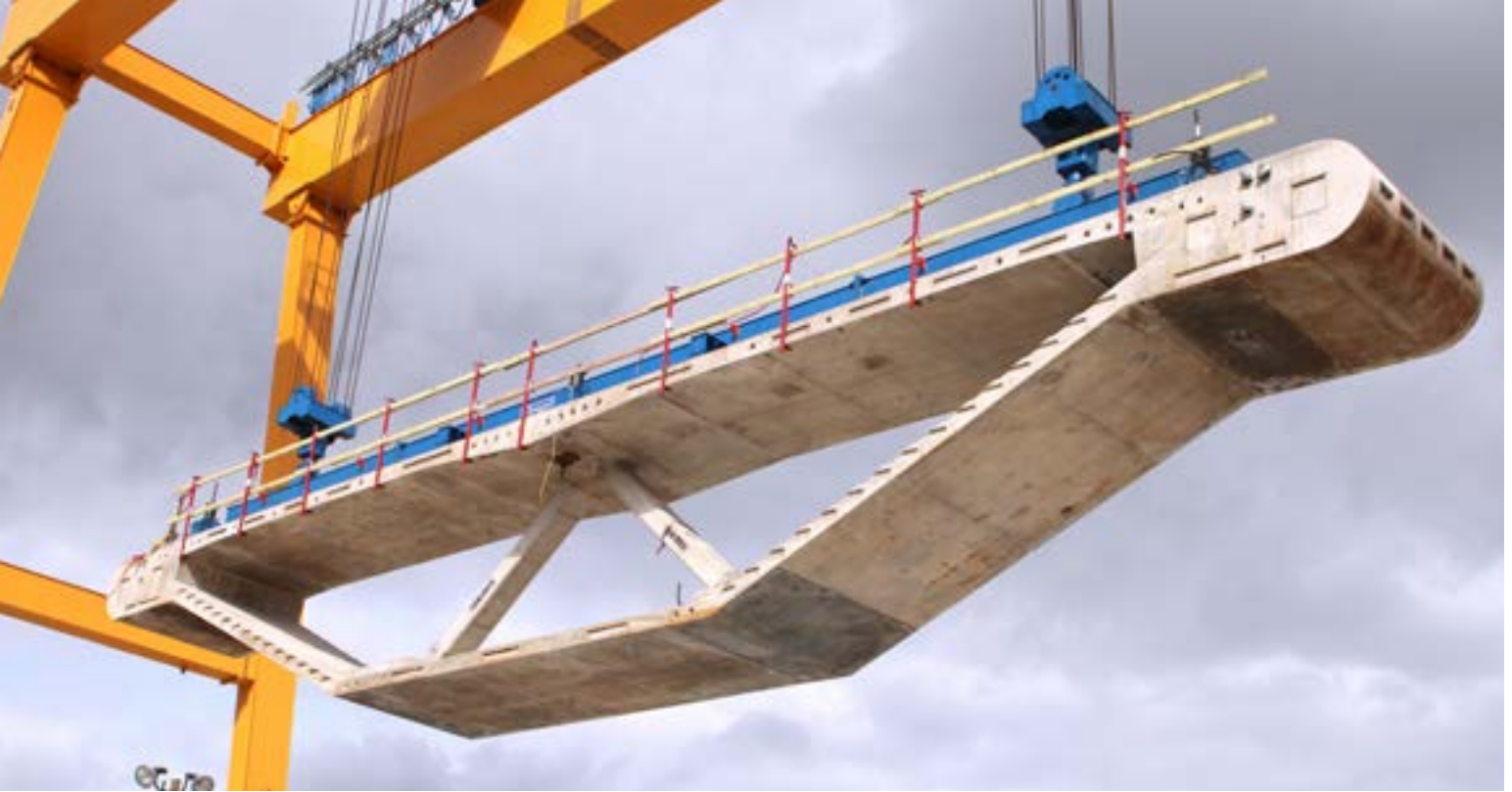
A completed precast segment is lifted from the long-line casting machine using a rail gantry crane.
