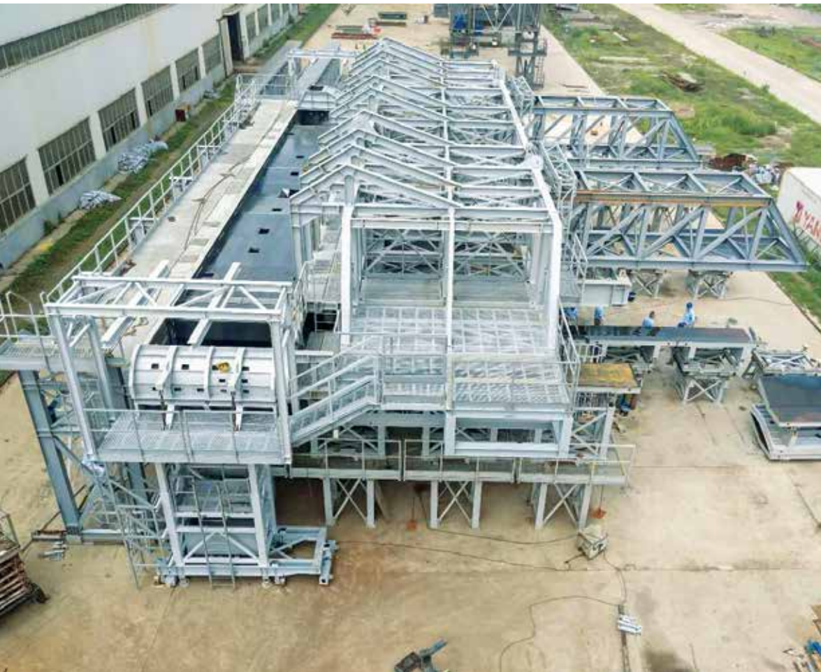
Long line segment casting machine under construction in China. (Photo courtesy of DEAL.)
