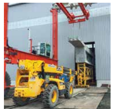
Pier segment loaded on skeleton soffit table then moved into building for match casting with typical cantilever segments, (Photo courtesy of FIGG.)
