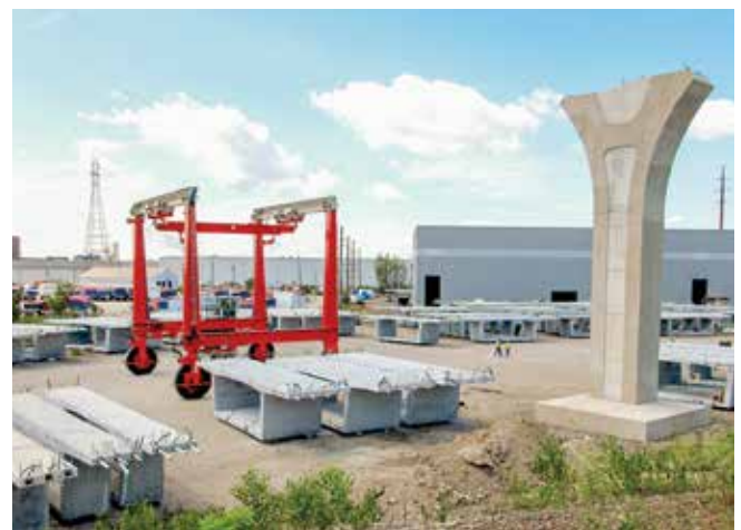
The casting facility is located adjacent to the bridge alignment in the existing right of way. As of September 28, 2018 29% of the 685 segments have been cast on site. (Photo courtesy of FIGG.)
