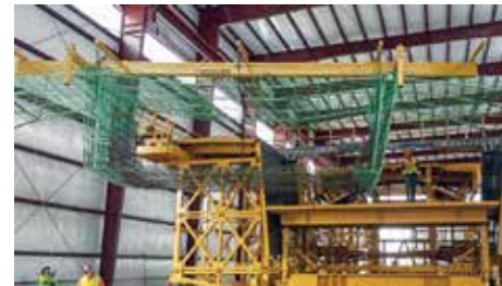
Loading cell #2 casting machine with pre-tied segment rebar cage, (Photo courtesy of FIGG.)
