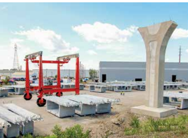
The segment reinforcement cages are pre-tied in temporary jigs outside the precast building and pushed on carts inside along an innovative rail system. (Photo courtesy of FIGG.)
