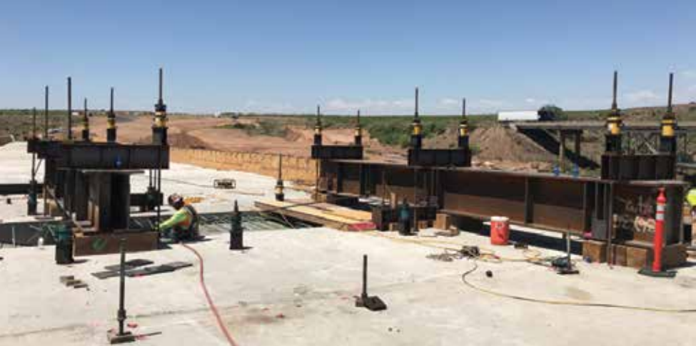
Closure beams were used to align and grade the cantilever tips and end spans for casting the closure sections. Photo: Malcolm International.
