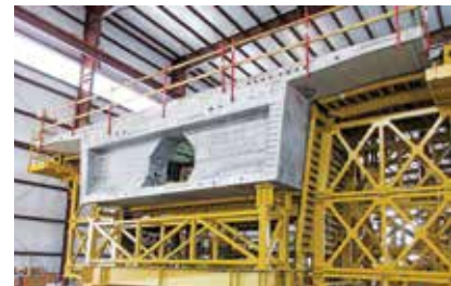
There are four total casting cells on the Cline Avenue Bridge project. Three cells are used to cast typical box girder segments inside a casting building that was erected for the project. (Photo courtesy of FIGG.)
