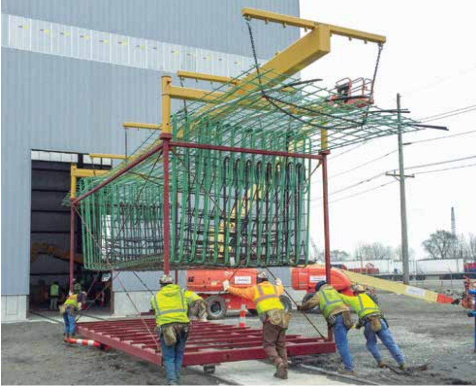
Crews rolling a typical reinforcement cage into building for precast superstructure segments. (Photo courtesy of FIGG)
