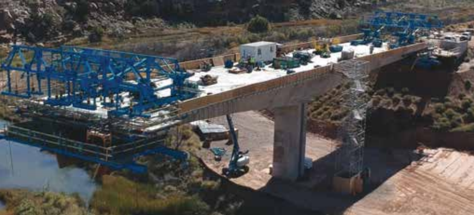
Form travelers at either end of cantilever 1. Geometry control and monitoring during segment casting ensured accurate vertical and horizontal alignments. Photo: Malcolm International.
