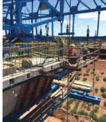
Formwork being set in preparation for casting the next box-girder segment. Photo: Malcolm International.
