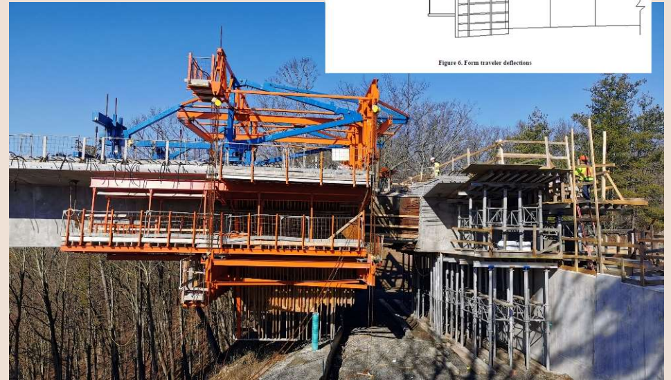
2 nd Critical stage – After concrete casting (finding out where the MFT 'landed')
