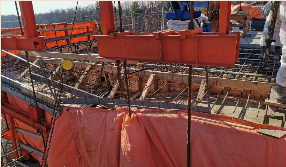
1 st Critical Stage – MFT Setup prior to concrete pour (assume MFT local deflection under wet concrete)
