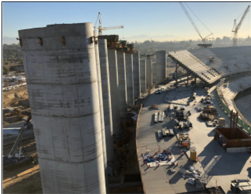
Figure 8.7 – SoFi Stadium Roof Support Columns, CA (Photo Courtesy of McNary Bergeron & Johannesen)
