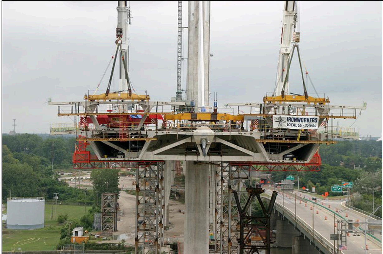
Figure 7.14 – Typical Anchor Block, Veterans’ Glass City Skyway, OH (Photo Courtesy of FIGG)
