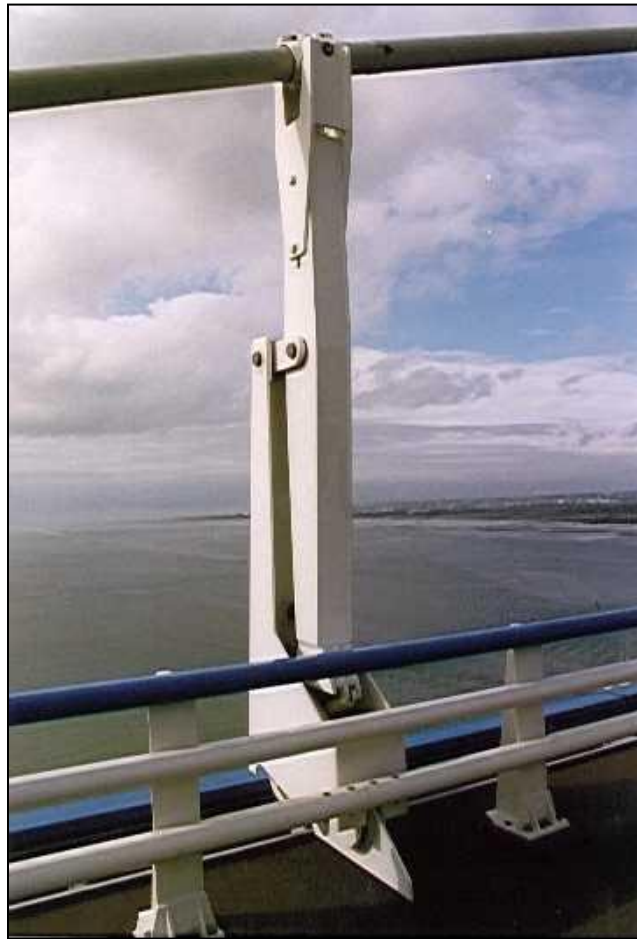
Figure 7.78 – Hydraulic Damper and Frame Connected to the Superstructure (Photo Courtesy of SYSTRA IBT)
