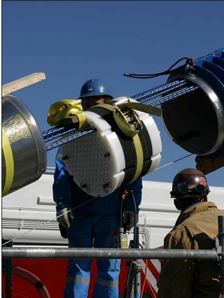
Figure 7.79 – HDPE Cheese Plate Inside the Stay Pipe at the Hydraulic Damper Connection (Photo Courtesy of FIGG)
